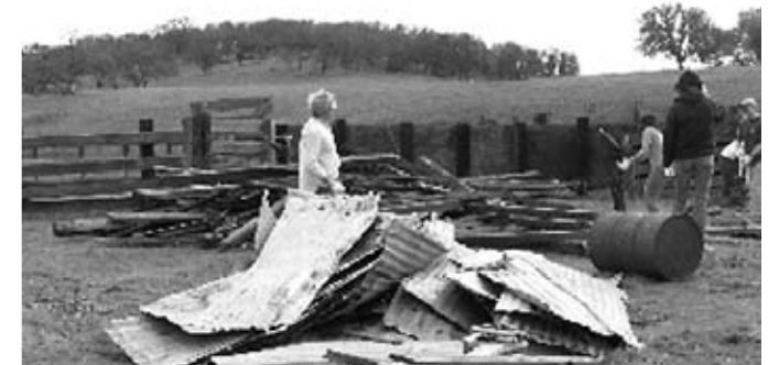
Granite Construction and Eagle Scout work hard at Deer Creek Hills Preserve.
